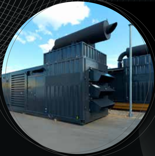
12 MW DIESEL POWER PLANT FOR RESERVING A DATA CENTER IN MOSCOW
