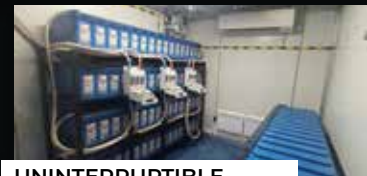
UNINTERRUPTIBLE POWER SUPPLY (UPS)
