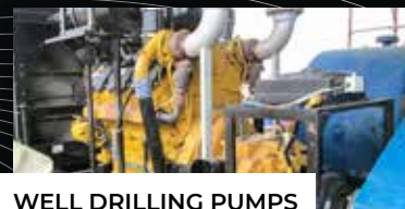
WELL DRILLING PUMPS
