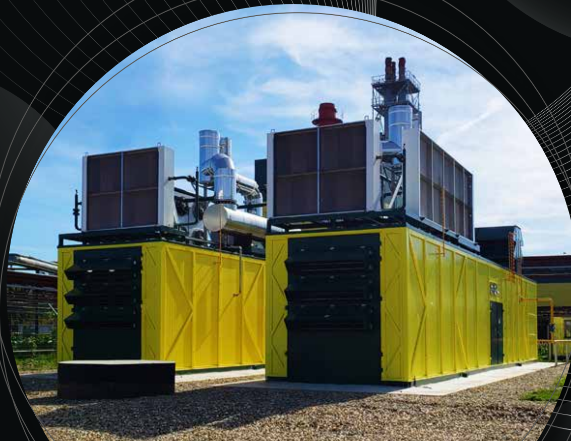
5.4 MW GAS POWER PLANT FOR THE INDUSTRIAL PARK «RODNIKI» IN THE IVANOVO REGION (RUSSIA)
